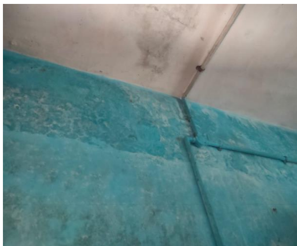
Image 3: Damp Walls in Semmenchery
