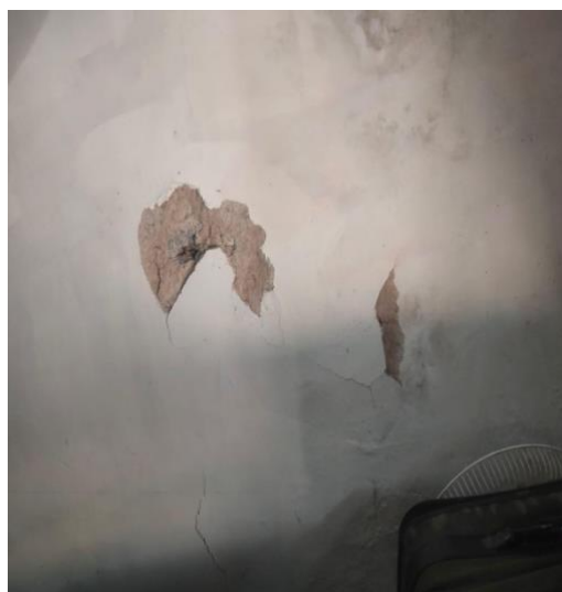
Image 2: Cracked Walls in Semmenchery
