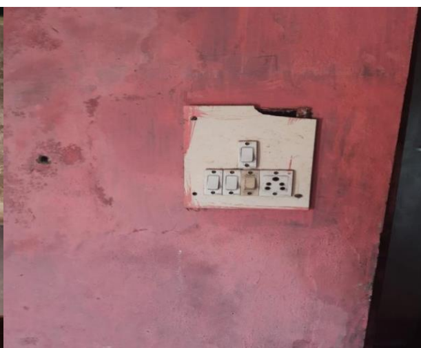
Image 6: Damp walls have affected electrical wiring resulting in electrical shock
