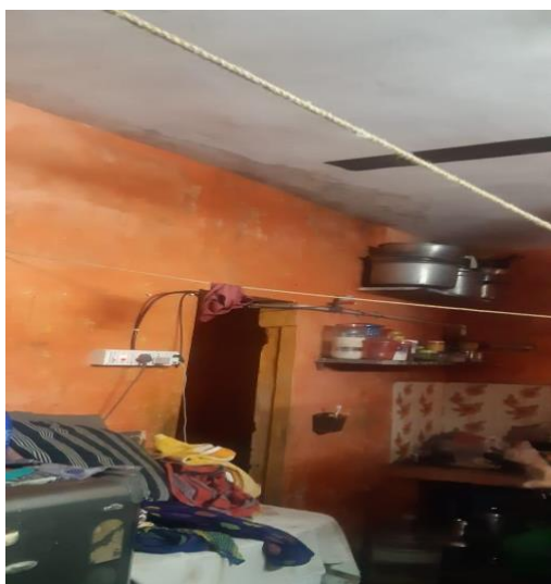
Image 1: Damp Walls in AIR Site
