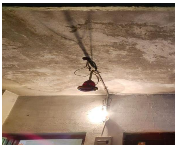
Image 5: Damp Ceiling in Perumbakkam
