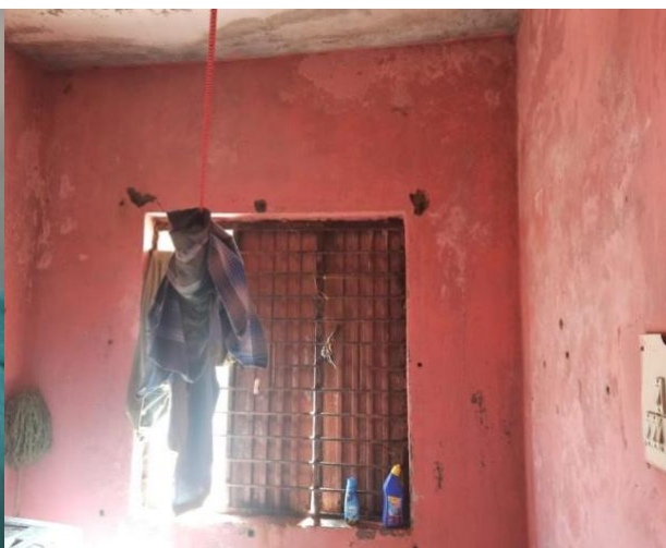
Image 4: Damp Walls in Perumbakkam
