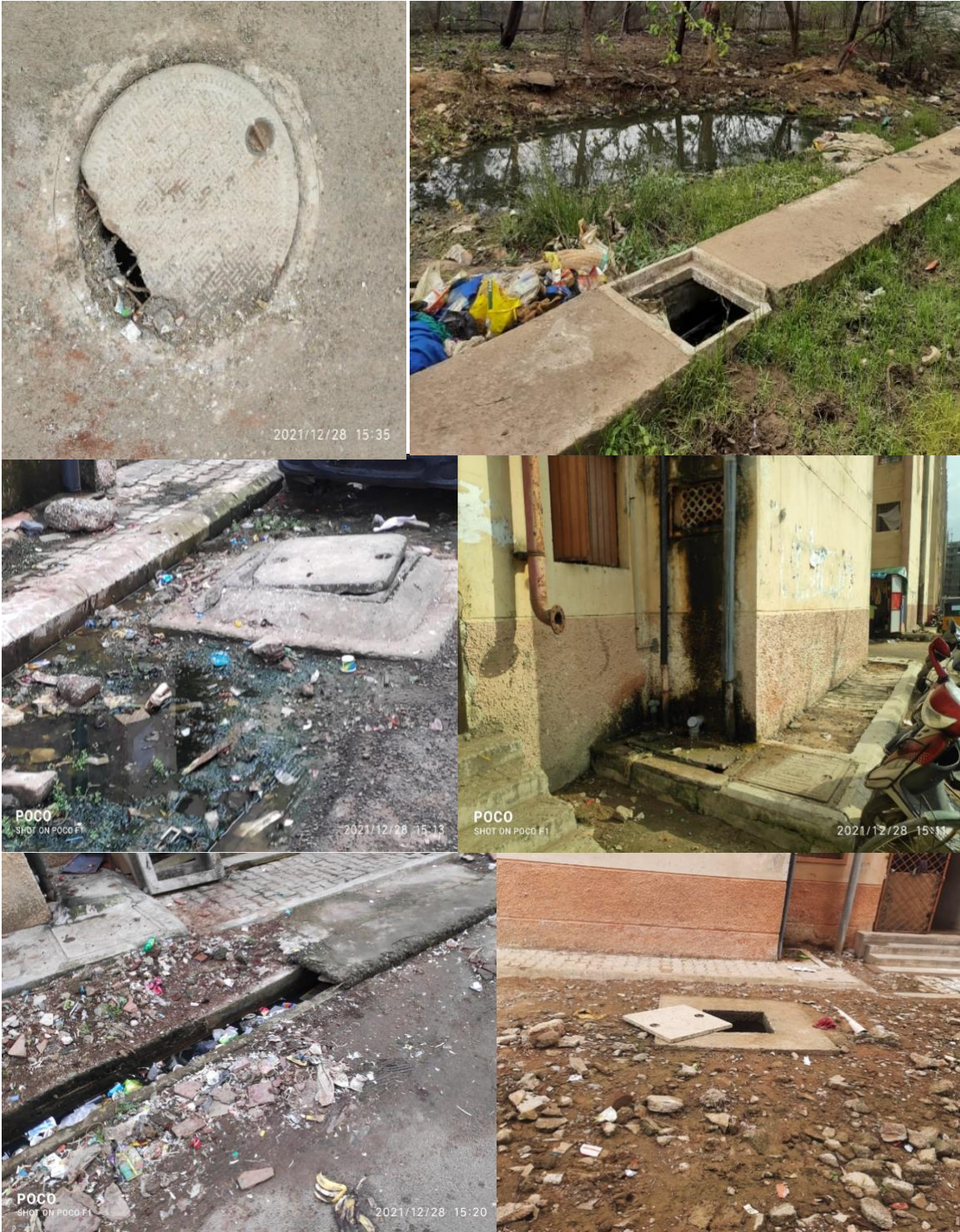
Image 22 to 27: Open Drains in Perumbakkam
